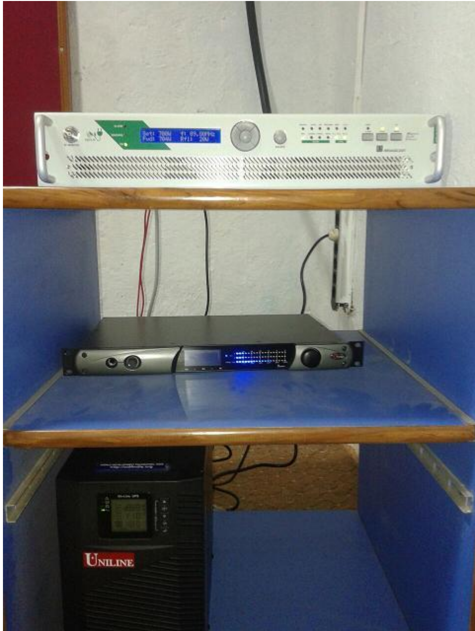
Transmitter and processor system (Common at all Places)
